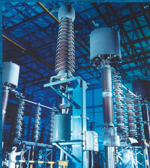
Peterhead Power Station
